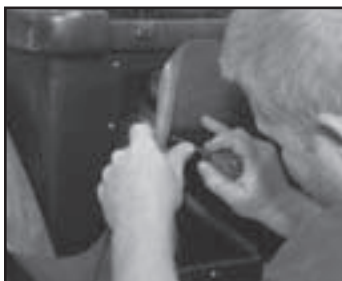
Fig. 13 Mark the outer perimeter of the skimmer opening on the liner; then mark a second box 1.5" inside of it. Cut out at inside mark.
