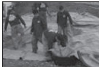
Fig. 6 Place the liner on top of the underlayment following the same installation procedures.
