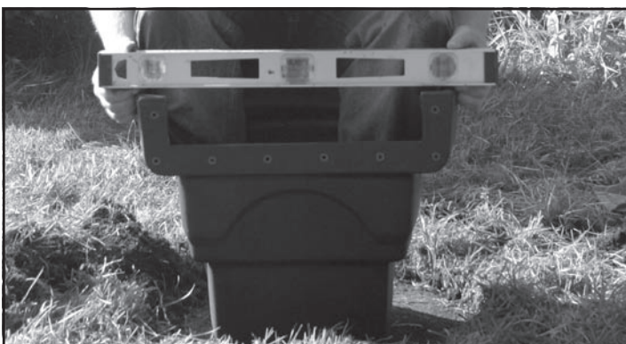
Fig. 3 Level the MicroFalls® filter side to side as well as front to back.
