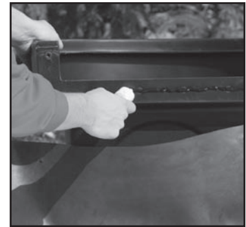
Fig. 8 Apply a thick bead of fish-safe silicone sealant around the MicroFalls® filter opening.
